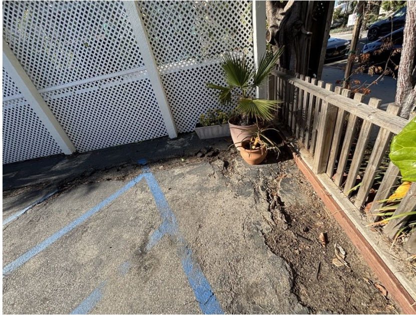
HC parking off Sanborn Ave. in need of repaving
