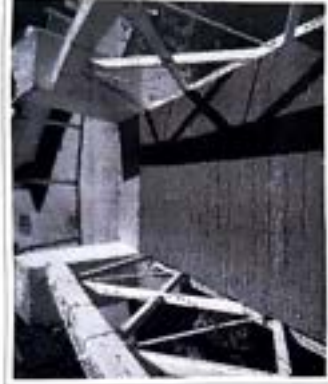
Photo 10: Full bridge overview showing overall deteriorated condition
