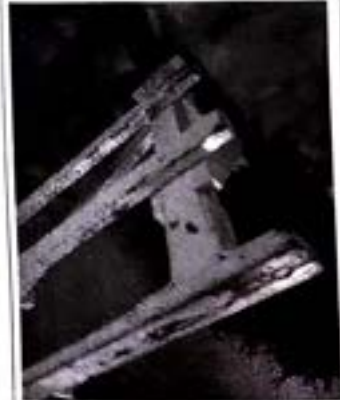
Photo 7: Severe paint loss throughout railing — bare wood exposed
