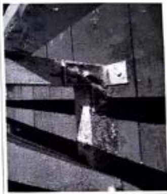
Photo 8: Microalgae at post bases where moisture accumulates
