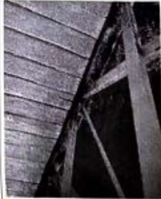
Photo 5: Dark mold growth along base stringer at waterline
