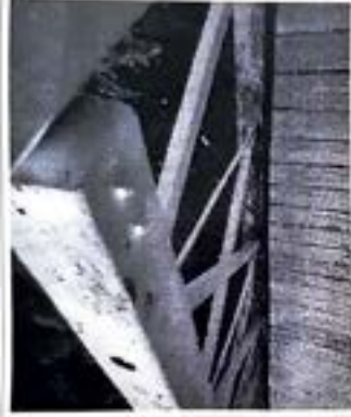
Photo 4: Paint crazing on rail cap, missing wood sections, exposed fasteners
