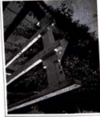
Photo 1. Weathered railing post — chipping paint, rusted hardware
