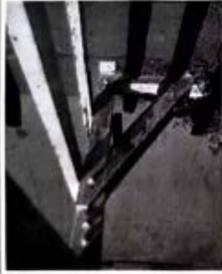
Photo 3: Heavy green algae/mold on structural bracing
