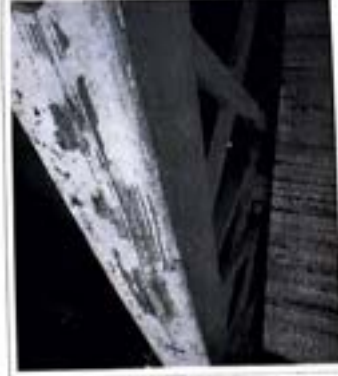
Photo 2. Extreme paint peeling on top rail — bare wood and mildew staining
