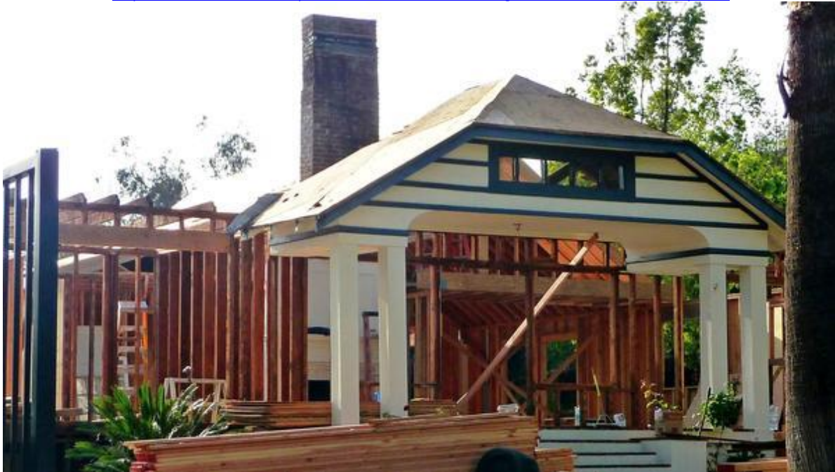
Only the porch and facade remain during a reconstruction of this 1930s Craftsman home, located in La Cañada Flintridge, on Feb. 7.
