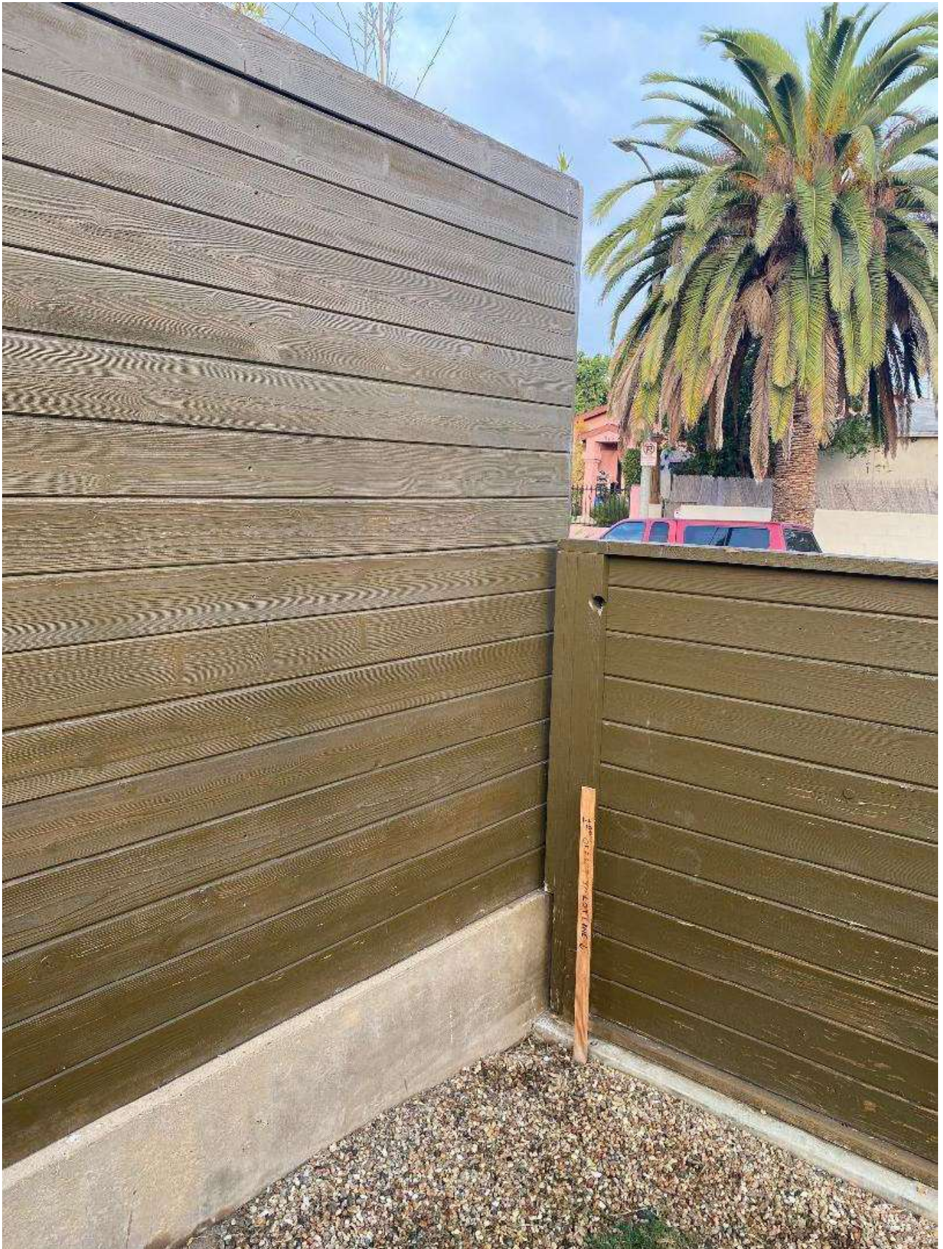
EXISTING FENCE BETWEEN 644-650 SUNSET AVE AND 652 SUNSET AVE TAKEN FROM 652 SUNSET AVE
