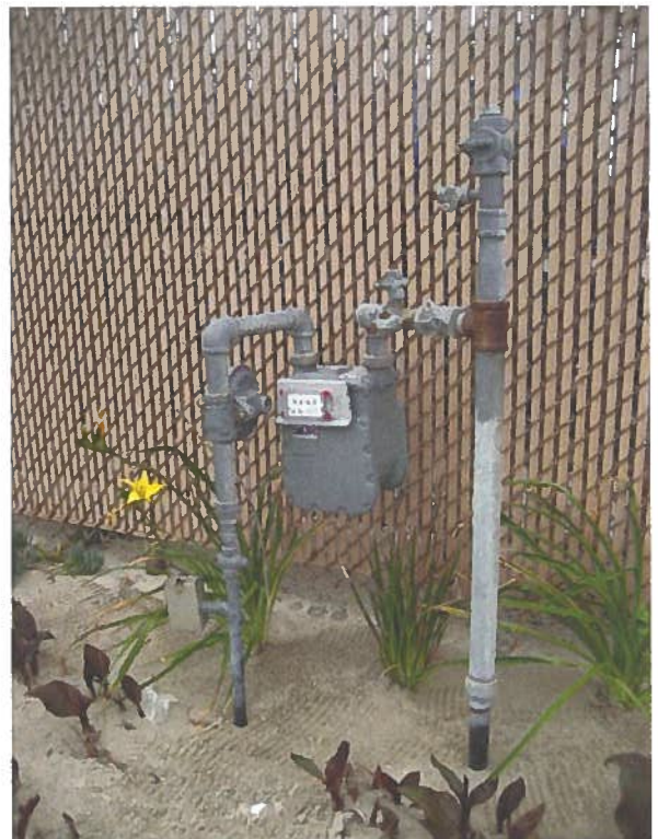
Existing gas meter missing seismic shut off valve
