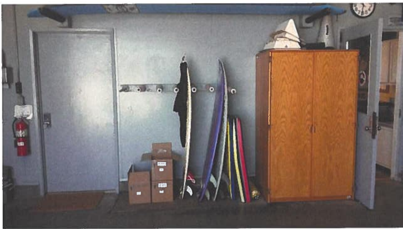
Toilet room facility-no accessible signage or accessible door hardware
