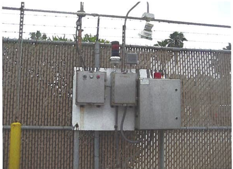
Existing fuel filling alarms and control panels
