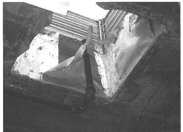
Existing fire sprinkler piping inside garage area
