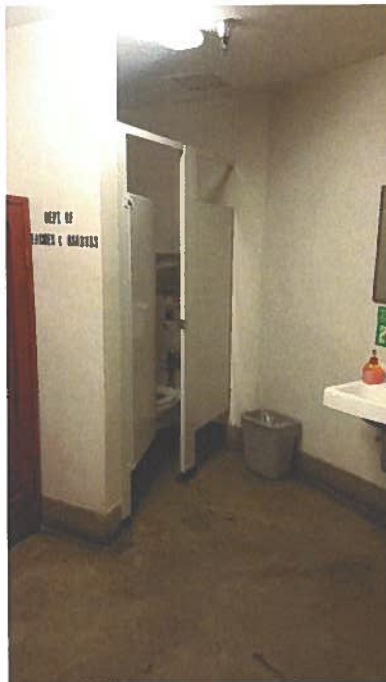
non-conforming toilet room design
