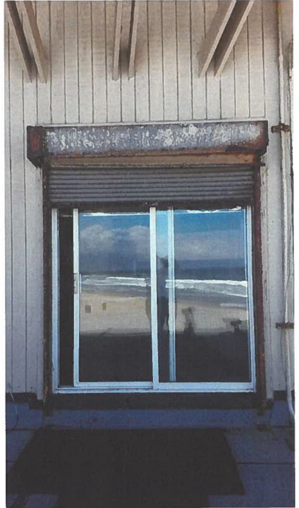
2 nd level rusted metal roll-up door shutter
