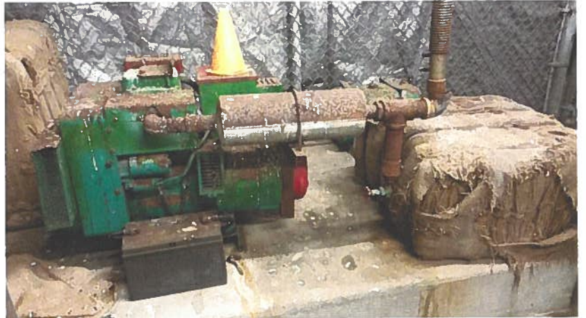
Existing Electrical Generator
