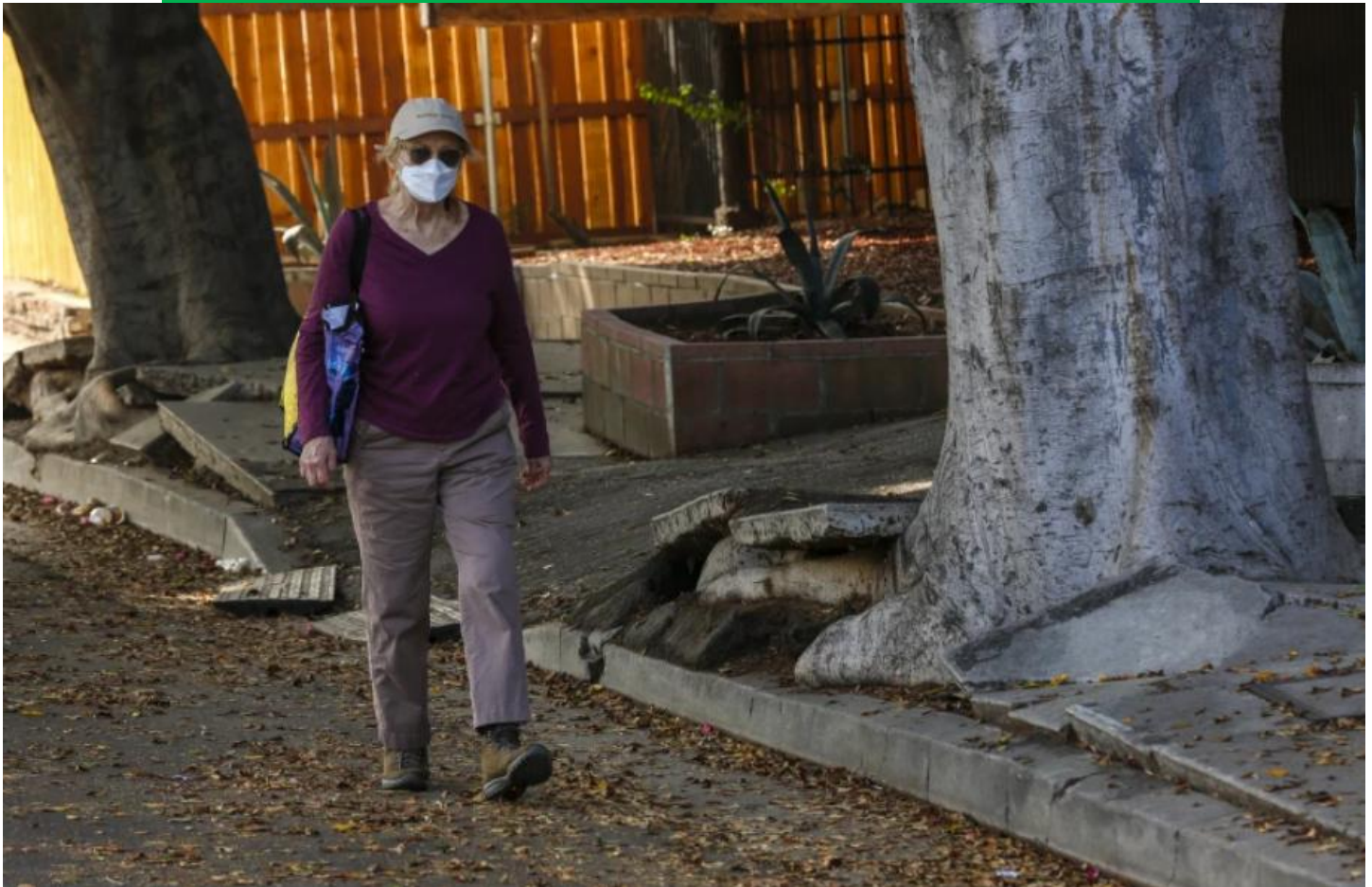
A pedestrian walks in the street to avoid a broken sidewalk on Griffith Park Boulevard in Silver Lake. (Irfan Khan / Los Angeles Times)
